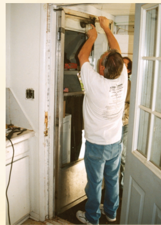
A Rebuilding Together volunteer repairs a broken screen door for an elderly homeowner.
